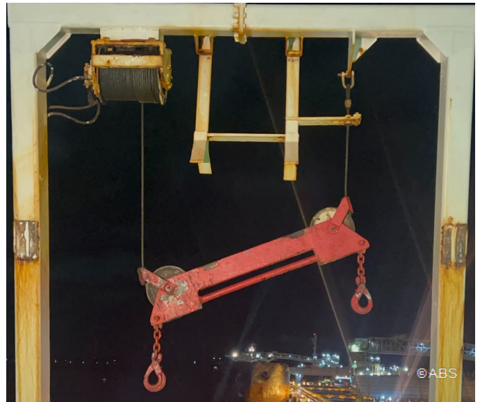
Freefall lifeboat recovery arrangement defective
