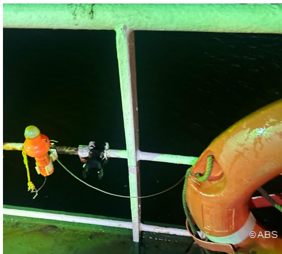
Lifebuoy self-igniting light malfunctioning
