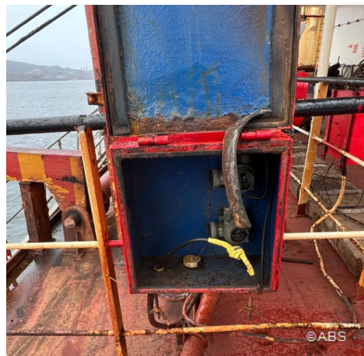
Electrical junction box, not maintained
