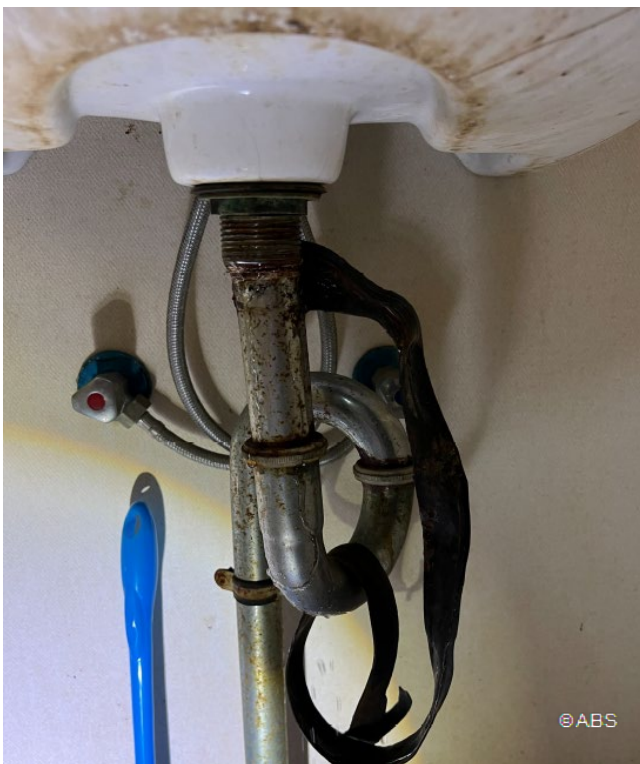
Accommodation sink, not maintained
