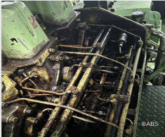
Generator engine fuel oil leakage points
