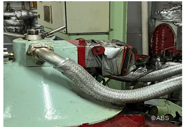
Heavy Fuel Oil Purifier connection with unapproved tape
