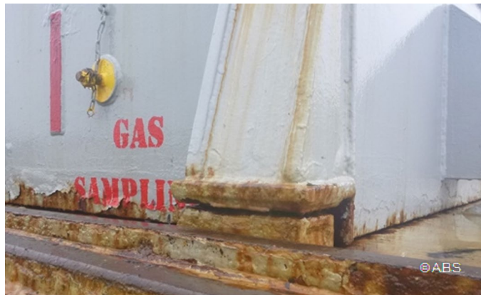
Hatch cover support pads with excessive wear, over compressed weathertight gasket and panels resting on coaming
