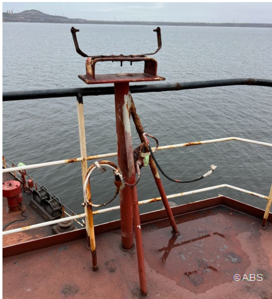
Flood light stand, not maintained
