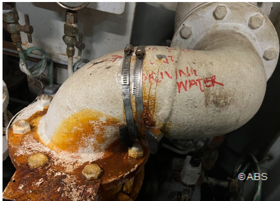
Ballast stripping pipe with soft patch strapped, leaking and not maintained
