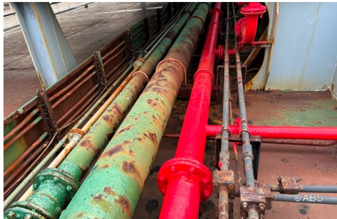
On deck, piping not maintained and wasted
