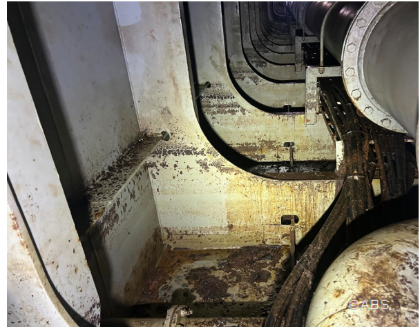
Sign of oil leakage in pipe trunk
